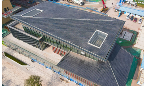
Location: Main Venue of CATL's World Energy Storage Conference Installed capacity: 97kW Application: Solar roof slate
