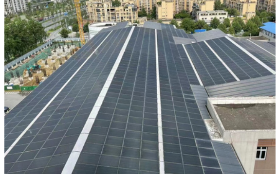
Location: Chengdu Pengzhou Hospital Project Installed capacity: 300kW Application: Solar roof tile
