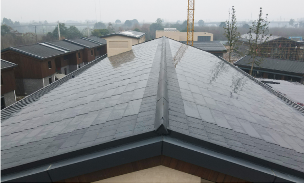
Location: Naked Hotel Project Installed capacity: 452.4kW Application: solar roof tile
