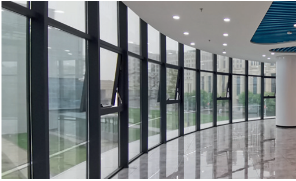
Location: BIPV Project for Western China Science And Technology Innovation Harbour Installed capacity: 226kW Application: Fixed window
