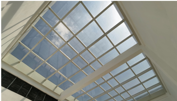
Location: Ruichang building materials sun room Installed capacity: 7kW Application: Skylight
