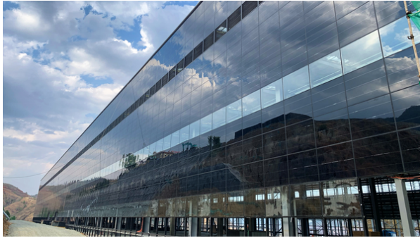
Location: Panzhihua Graphite Carbon Industrial Park Installed capacity: 1.25MW Application: Glass Curtain Wall
